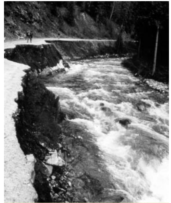
Roads constructed adjacent to rivers can threaten water quality and are prime candidates for removal.
